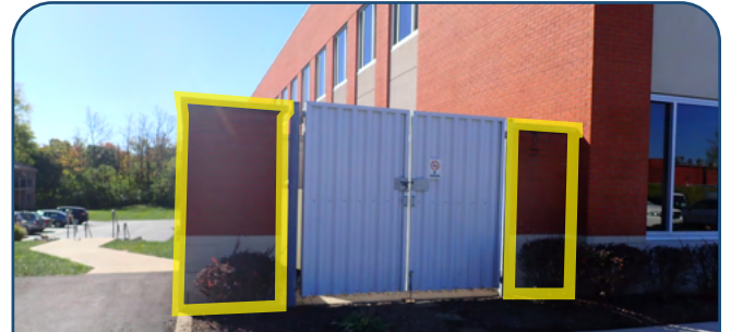
The screening of this mechanical equipment complements the design of the primary building, helping maintain the overall character of the development.
